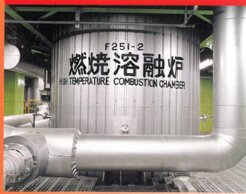
燃焼溶融炉 High Temperature Combustion Chamber
