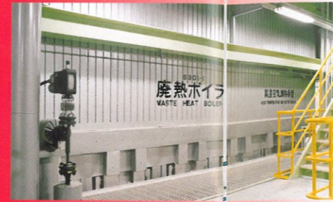
廃熱ボイラ(左)と高温空気加熱器(右) Waste Heat Boiler (left) and High Temperature Air Heater (right)
