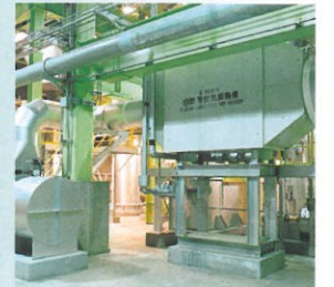
白煙防止装置 Flue Gas Reheating Facility
