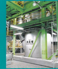
減温塔 Flue Gas Cooler
